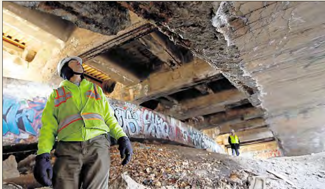
In crisis: Civil engineer Harry Smeltzer checks the crumbling, 96-year-old Heth's Run Bridge, an underfunded project in Pennsylvania that has lost out on $392 million in road spending because of "orphan earmarks."
